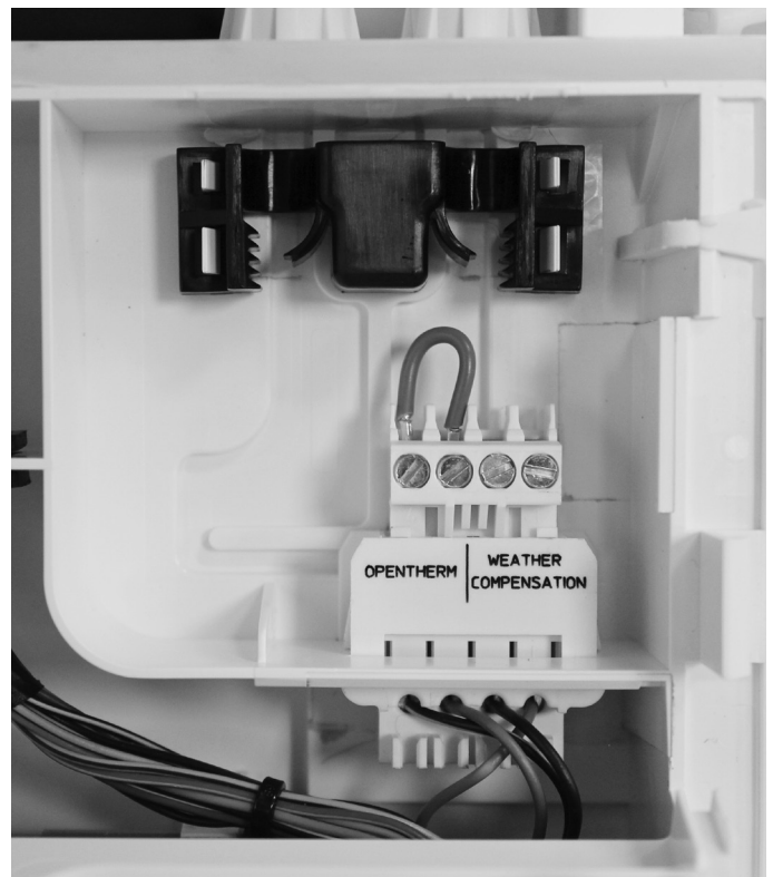
INSTALLER CONNECTIONS (RHS)
